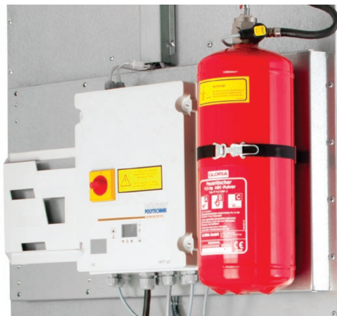
Fig. below: PLC-control, automatic fire extinguishing system
