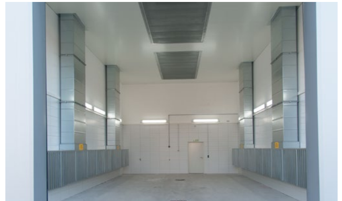
Wash cabin for paint preparation, 12 m x 7 m x 6.8 m with aeration.
